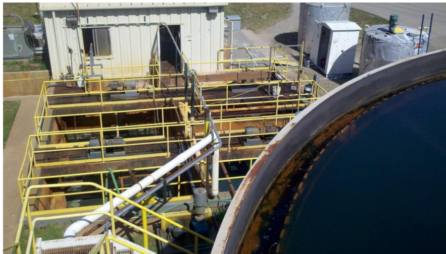
Figure 3: MPC Wastewater Treatment Plant prior to starting the trial. Note the control cells to the left, the overloaded Claricone at bottom right, trial tanks and control shelter supplied by Martin Marietta for receiving trailers, storage and pH-controlled metering of FloMag® H magnesium hydroxide slurry during the trial – located at top right.
