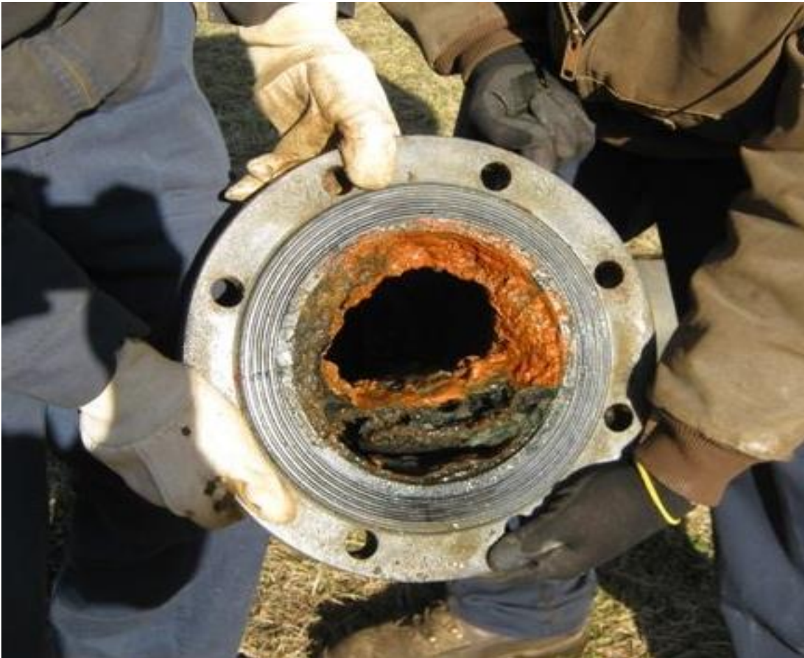
Figure 1: Gypsum sludge fouled the process when using lime alone to treat sulfuric acid wastewater. This problem has been eliminated with a combination of magnesium hydroxide slurry and lime.
